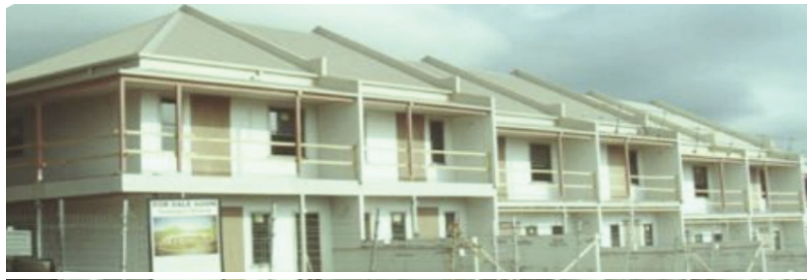
Figure 4: Eleven two storey units were built by only four workers in just five and a half weeks using GFRG technology.
